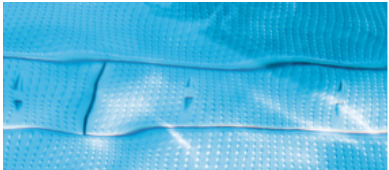
Treated water flows into the pool through jets in channels on the floor.
