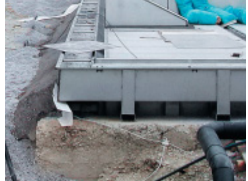
The new overflow gutter sits on the walls of the old pool.
