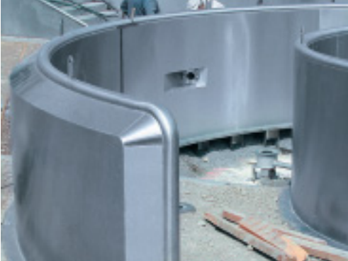
Stainless steel used for the self-supporting walls of the 'lazy river'.
