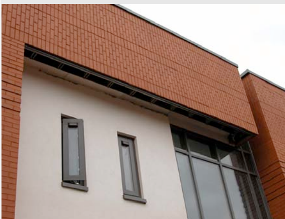
Figure 5: Construction of vertically stack bonded brickwork held up by masonry support system
