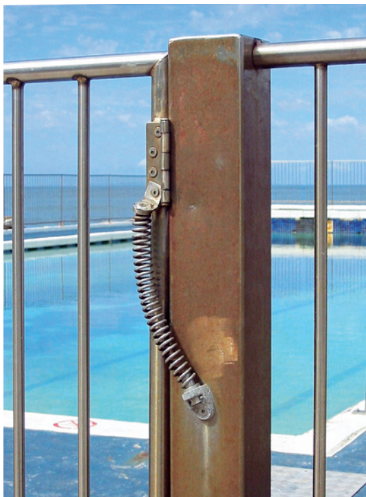
Figure B The contrast in appearance between the gate and support post is due to stainless steel chemistry and surface roughness differences. The corrosion-free gate is Type 316 stainless steel and the post that is discolored by corrosion is Type 304 stainless steel. (Photo Courtesy of Australian Stainless Steel Development Association)
