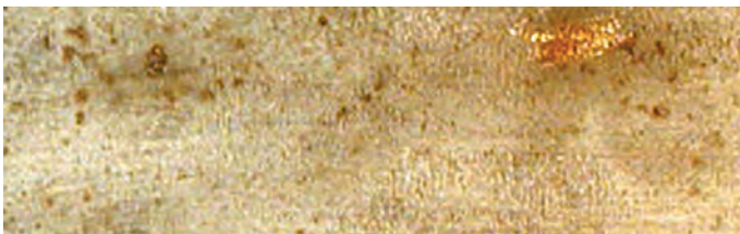
Figure B Sheltered Type 304 stainless steel components like this light pole will corrode in most coastal applications unless they are cleaned frequently. Monthly cleaning may be necessary. (Photo Courtesy of TMR Stainless)
