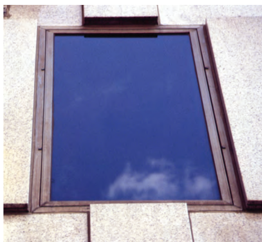
Figure C This Type 304 stainless steel window frame has not been cleaned in five years. Type 304 that is exposed to deicing salt must be cleaned regularly to remove corrosive deposits. Even with that precaution, some staining may occur between cleanings. (Photo Courtesy of the Nickel Institute)
