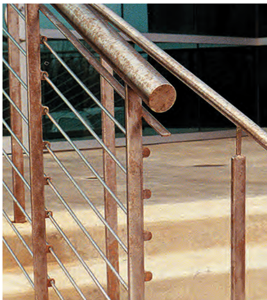
Figure B Type 304 stainless steel with a rough finish was the wrong choice for handrails exposed to deicing salt laden road mist. Cleaning will remove the staining but it will reappear every year. (Photo Courtesy of TMR Stainless)
