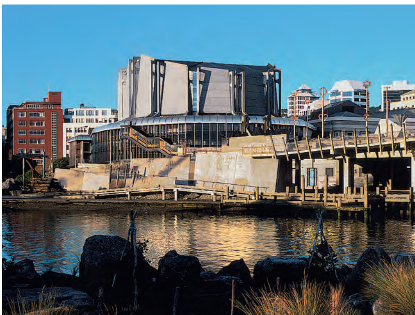
Figure A This image shows the building's original appearance in 1985 and its close proximity to the bay. Photo courtesy of the Nickel Institute.
