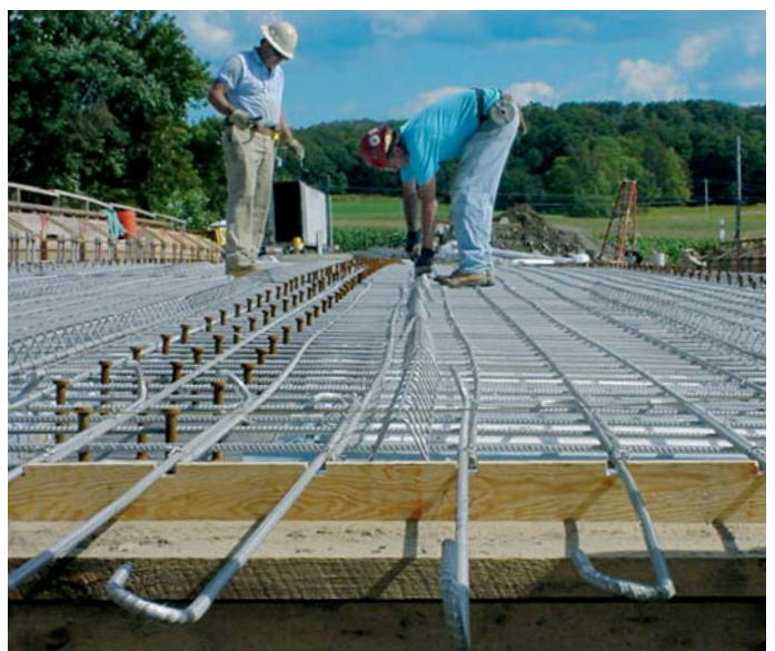
Installation of stainless steel rebar at the French Creek Bridge, Chautauqua Co., NY. (Photo Courtesy of Dunkirk Specialty Steel)
