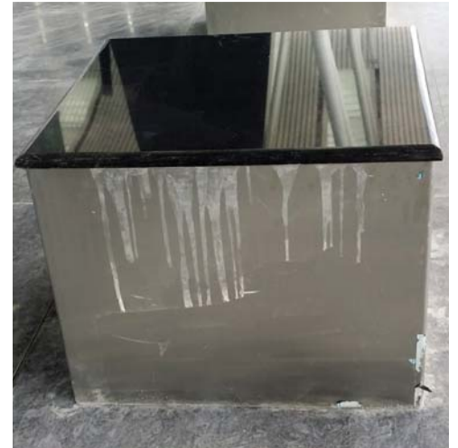
Figure 10. Outside an Indian airport, concrete spilled off the sides of these bollards when they were filled. Unfortunately, it was not washed off immediately. Power-washing may be effective in removing the deposit.
