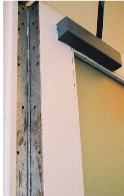
Figure 3. A maintenance worker 'cleaned' the hinges in this natatorium room with a household carbon steel wool pad. The corrosion is from the resultant embedded iron particles.
