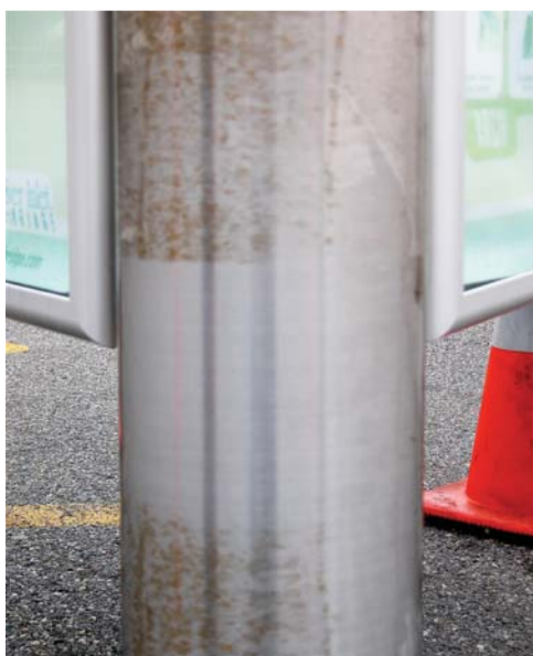
Figure 8. This pipe supports a beach park canopy. Unfortunately, the supplier did not use an ultraviolet-rated strippable film, and the pipe was exposed to the sun for several days prior to the removal. The areas with residual adhesive accumulated far more coastal salt than surrounding surfaces, causing light surface corrosion. It was removed with fine abrasive paste suitable for cleaning glass and is now performing well. The test area is shown.
