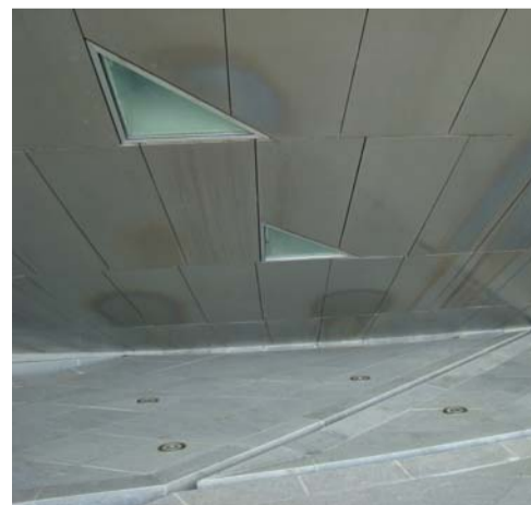
Figure 2. This Chinese museum has a fountain along one side, which sprays water on to the surface. The water's high total dissolved solids (TDS) content is causing staining on both the stainless steel panels and the stone. While this staining can be removed, avoiding the problem by installing a reverse-osmosis (RO) system is best.
