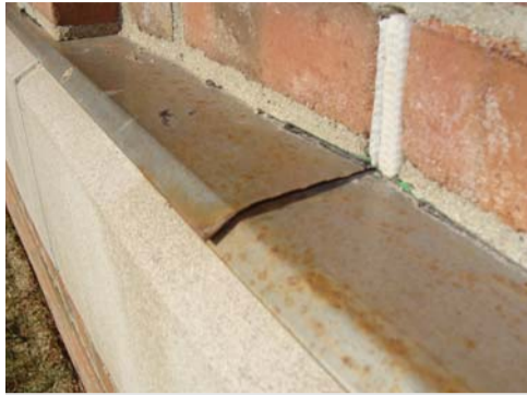
Figure 7. Muriatic (i.e., hydrochloric) acid was used to clean the masonry, causing corrosion of the drip edge. Similar damage has been observed by this author on kitchen cabinets after interior tile cleaning and on exterior railings and doors after concrete cleaning.
