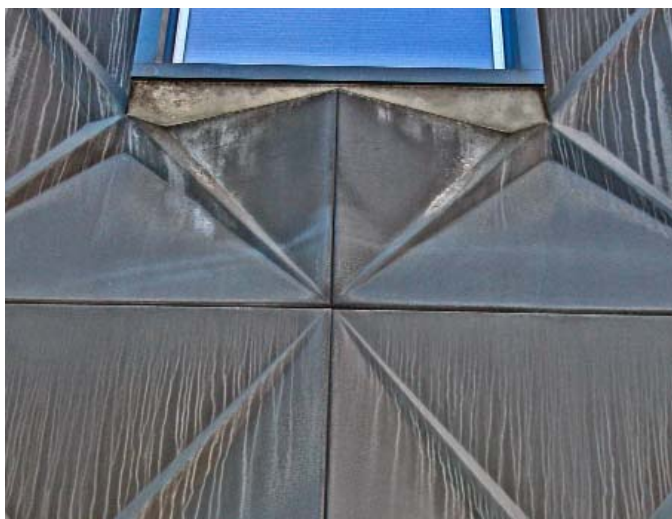
Figure 4: Deicing salt corrosion of anodized aluminum panels on the second floor of an office building
