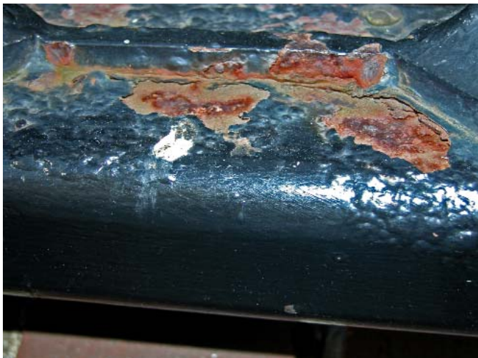
Figure 7: As evidenced by the surface “bubbling” of the paint, this carbon steel coating failure is accelerating the corrosion rate. Moisture and corrosive substances are getting under the coating edges creating crevice corrosion. More frequent paint removal and repainting are necessary to extend service life.
