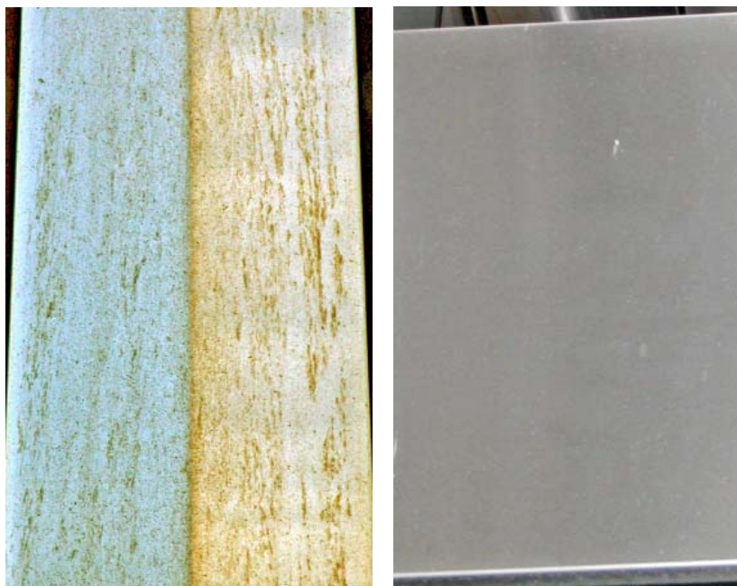
Figure 9: Both stainless steel panels are on the second floor of nearby buildings and are exposed to deicing salt. Neither has been cleaned and dirt and some residual salt was visible. The Type 304 panel (left) is exhibiting superficial corrosion staining while the Type 316 panel (right) remains corrosion free.
