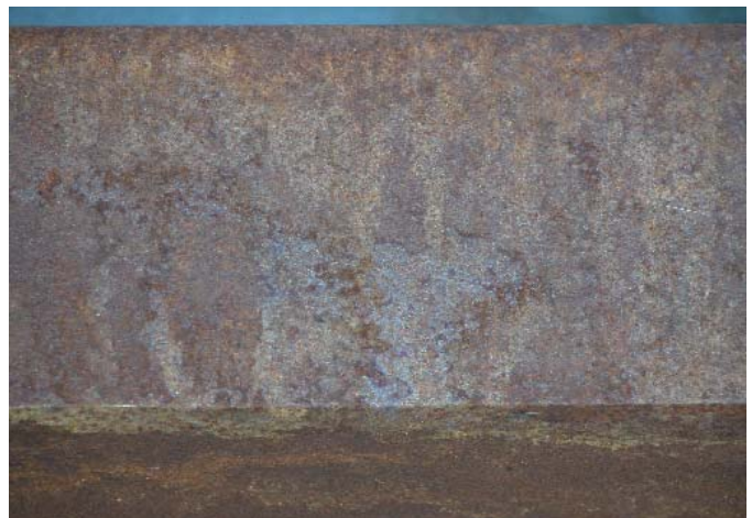
Figure 8: Weathering steel with deicing salt damage on a building exterior.
