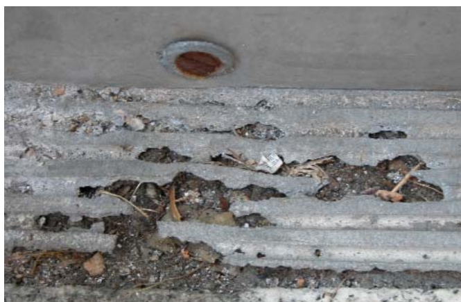
Figure 3: Severe deicing salt corrosion of an aluminum door threshold
