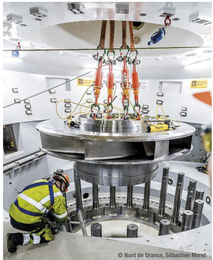
➤ Installation of a pump turbine. The turbine blades are made of martensitic stainless steel, containing 0.3–1.0% molybdenum.
