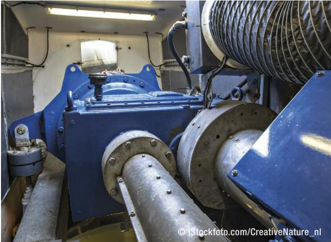
➤ The interior of a wind turbine nacelle with drivetrain.
