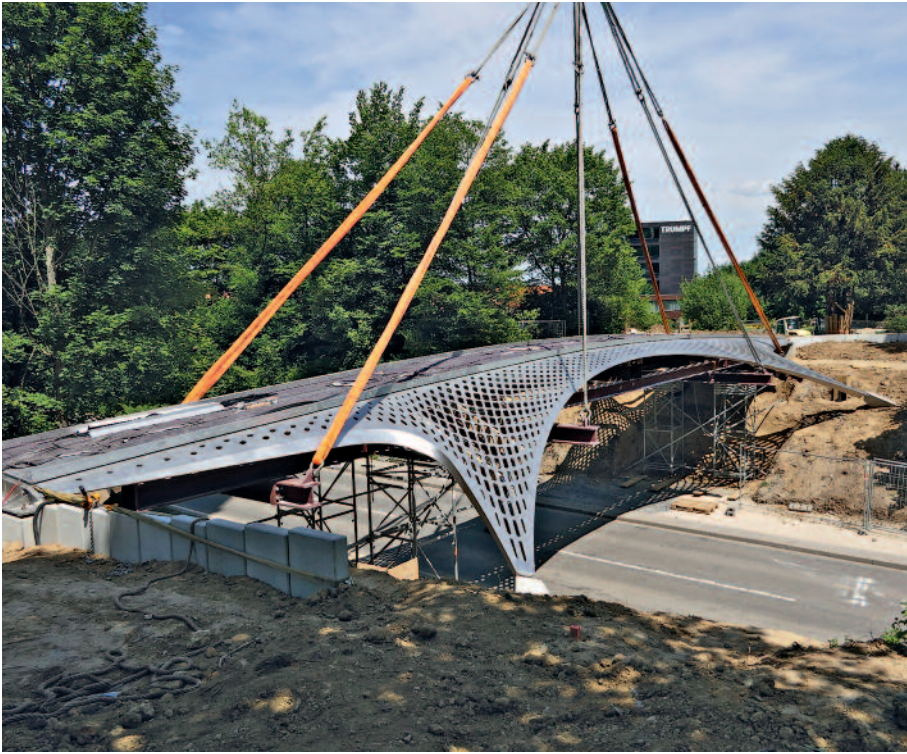
The bridge being lowered into its final position by crane; it is only self-supporting once placed in this exact position. © schlaich bergemann partner
