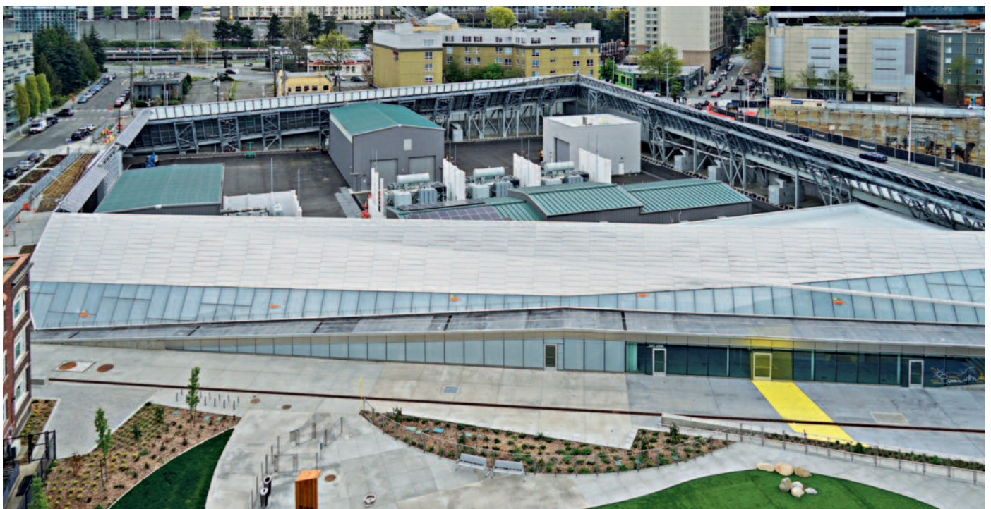
An aerial view of the substation prior to opening to the public in July 2019. © Seattle City Light
