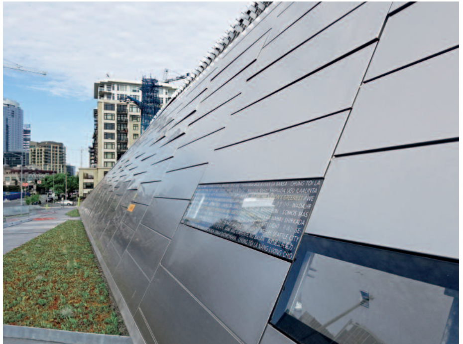
A closer look at the substation's stainless steel panels. © Seattle City Light
