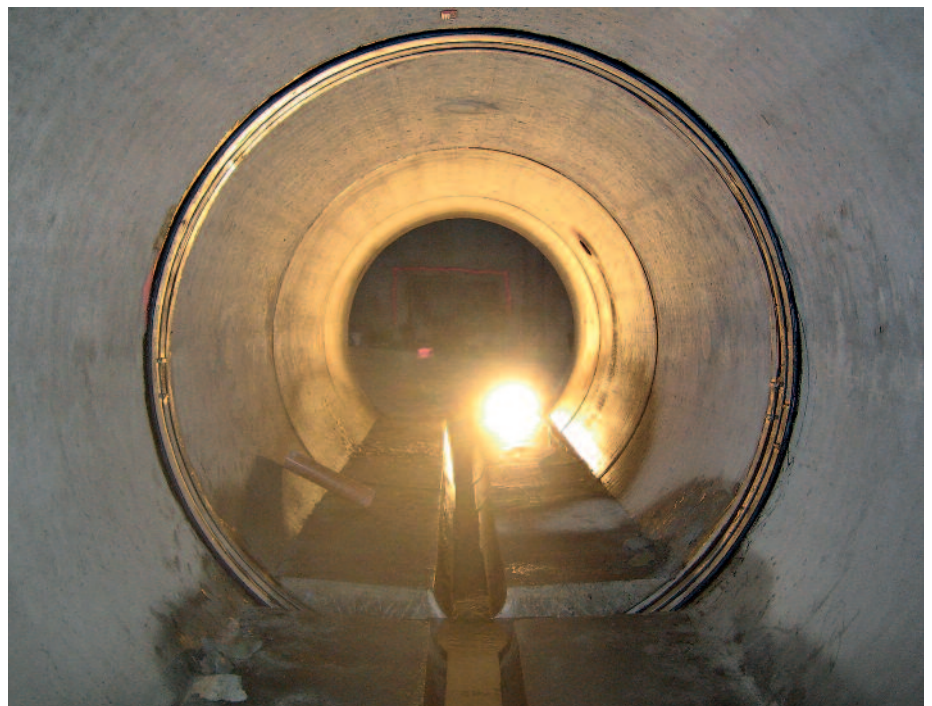
The inside of a large diameter pipe repaired with the sealing system. © AMEX
