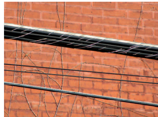
Communication cables firmly lashed to messenger wires strung along the side of a building.
