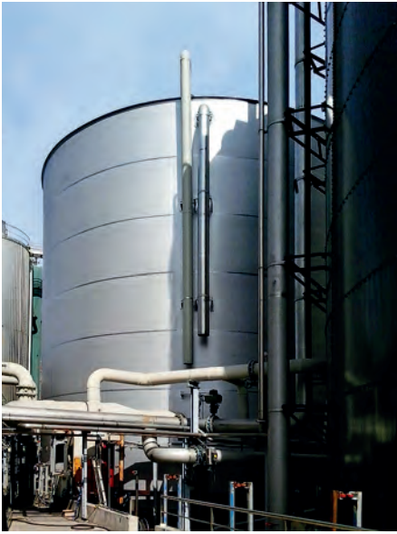
A 2205 stainless steel tank at a brewery in Spain. © Outokumpu
