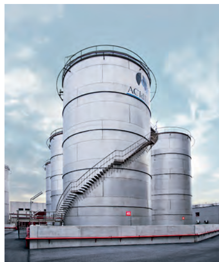
2304 duplex stainless steel tanks at the tank terminal in Bilbao, Spain. © Outokumpu/Acedika
