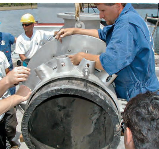
Technicians are reviewing the steps required to install the sleeve correctly. © Charleston Commissioners of Public Works
