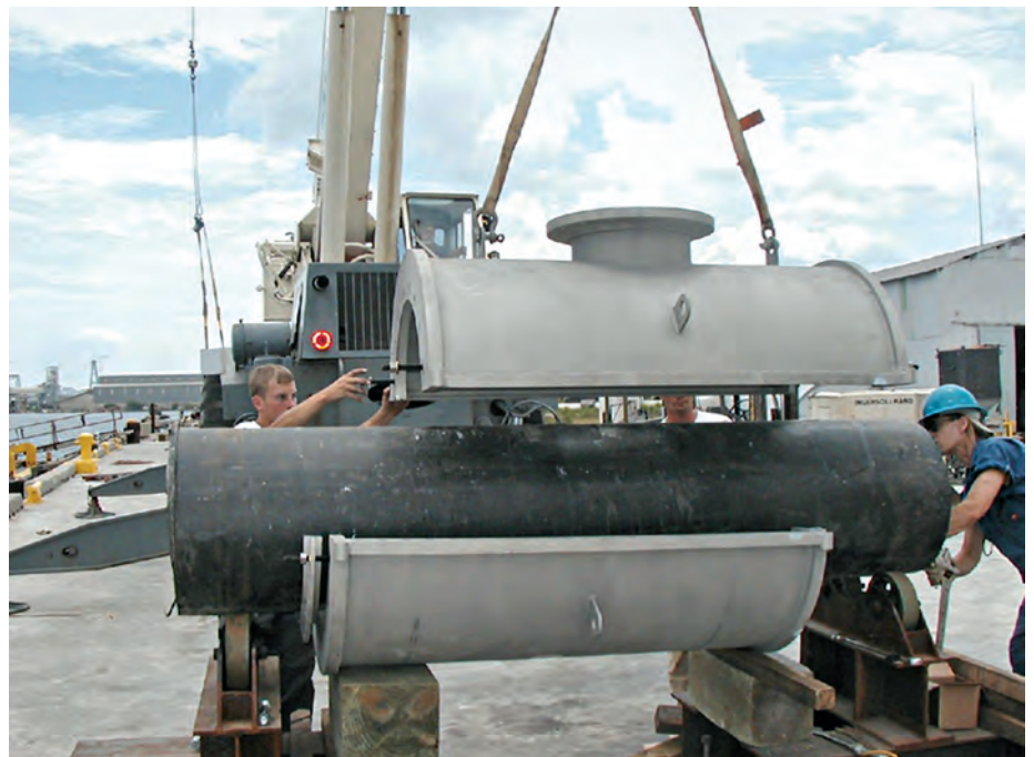
"Mock" installation of a custom-fabricated Type 316 stainless steel repair sleeve. The technicians are practicing the underwater installation on a piece of pipe in the dry. © Charleston Commissioners of Public Works
