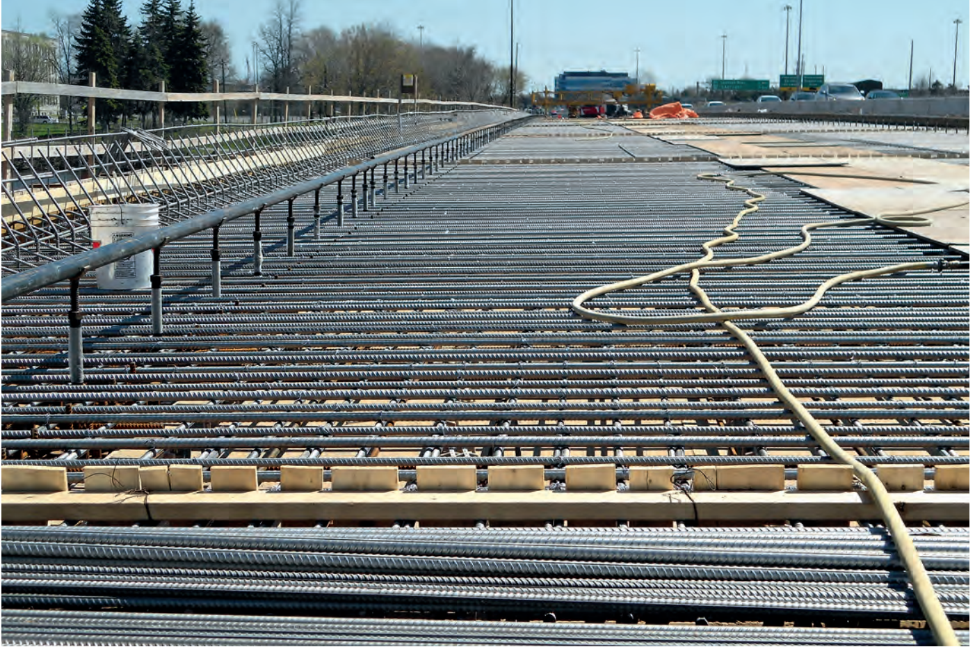
Stainless steel rebar installation on the Hurdman Bridge in Ottawa. The work is done in stages so that some traffic can continue to flow across the bridge as seen in the background of the picture. © Frank Smith
