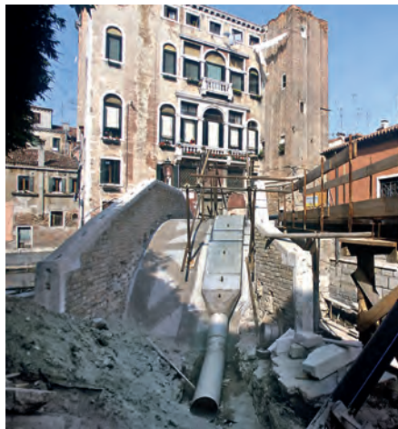
Installation of a flat stainless steel duct for water and gas services on the San Boldo bridge. © Daniele Resini for Insula spa, municipal agency for the urban maintenance of Venice.
