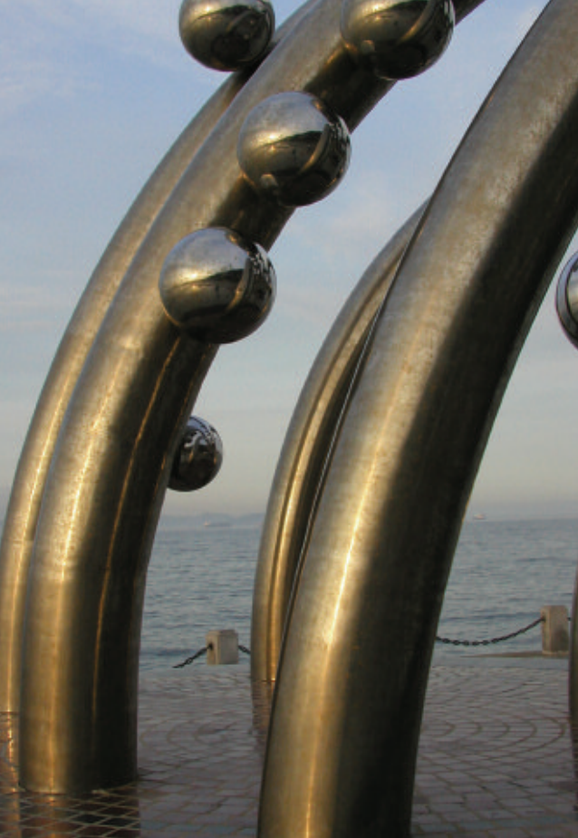
Figure 3: Corrosion staining on stainless steel due to incorrect grade selection in a demanding environment
