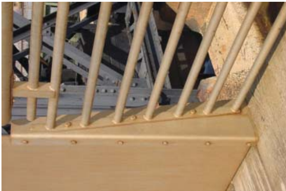
Figure 3. A reddish stain was evident on the 316L railing and panel adjacent to the pier wall, which is frequently splashed by the impinging waves caused by river vessel traffic. The evaporative concentration of salt and chlorides on the surface of the stainless steel results in an aggressive, corrosive environment.
