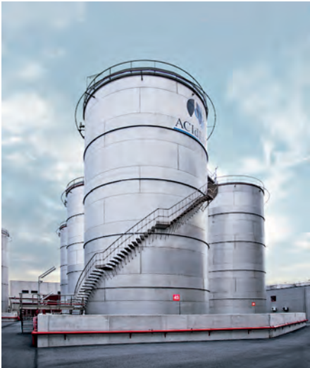
2304 duplex stainless steel tanks at the tank terminal in Bilbao, Spain. © Outokumpu/Acedika
