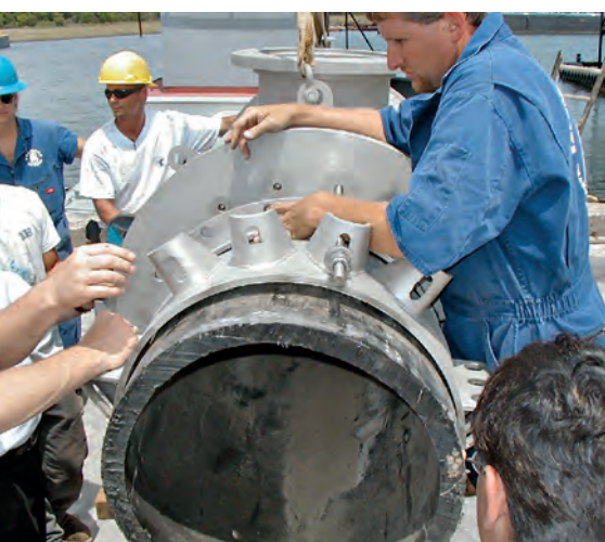
Technicians are reviewing the steps required to install the sleeve correctly. © Charleston Commissioners of Public Works
