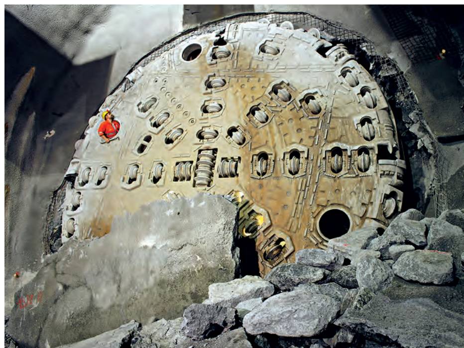
Cutter head after break-through in one of the Gotthard tunnel pipes. Photo: Herrenknecht AG
