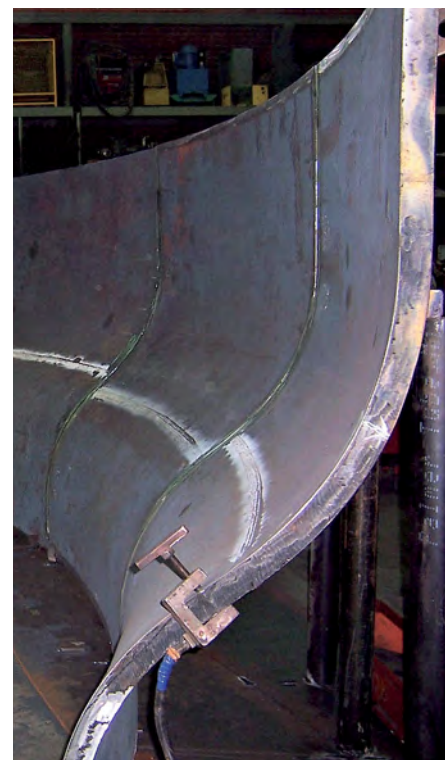
Pre-assembly of the knuckle ring at BlueScope Steel’s Port Kembla Steelworks. Photo: BlueScope Steel.
