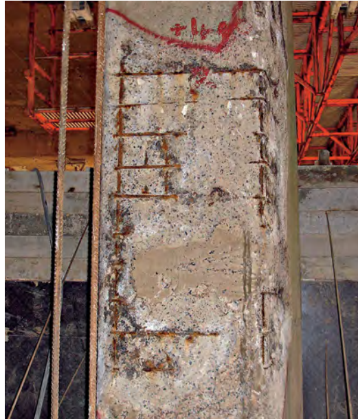
The maritime environment had taken a toll on the mosque’s ocean-front portions, leading to deterioration of the pillars under the prayer room. Photo: Ugitech.
