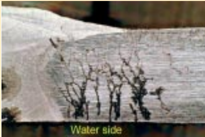
Figure 3 Macro-photograph of chloride stress corrosion cracking (CSCC) in the base plate adjacent to the vertical weld, showing classic, branched, intergranular morphology and growth from the internal surface outwards
