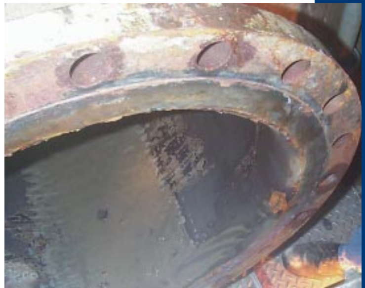
Figure 1: Lined carbon steel spool piece from intake structure. Significant corrosion can be observed on the edges of the pipe, where the lining has imperfections.
