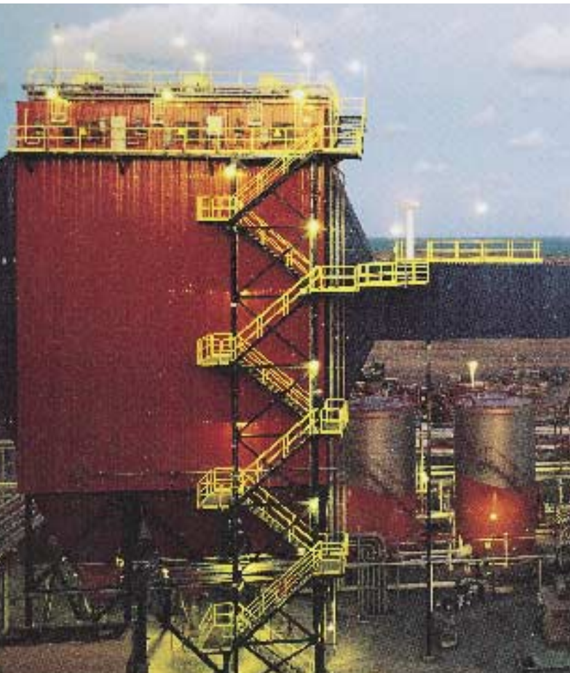
Seawater-based flue-gas desulphurisation plant
