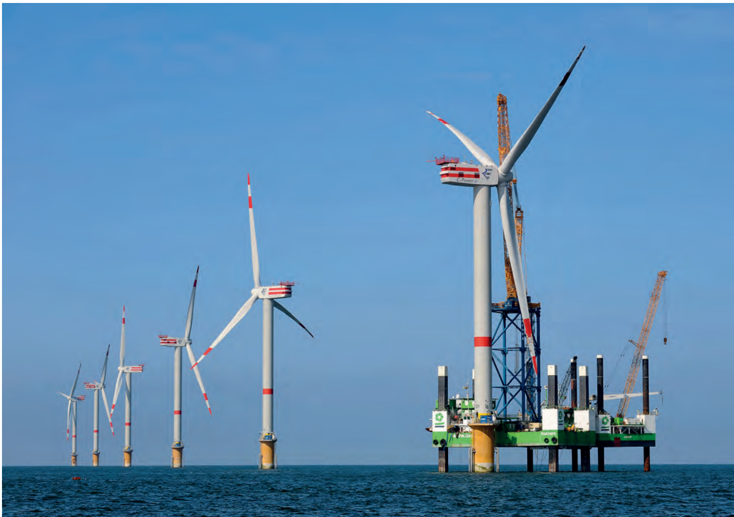
Figure 9. Installation of 5 MW offshore windmills in the Thornton Bank project, Belgium; foreground: jack-up platform with hoisting cranes (courtesy Jan Oelker).
