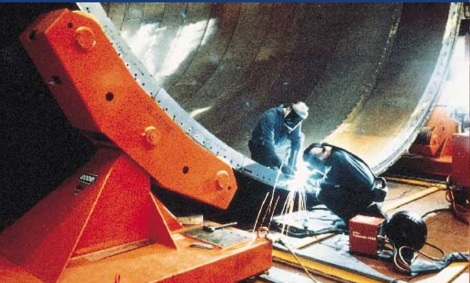
Clean gas ducting for Flue Gas Desulphurisation plant at the National Power, Drax Power Station. Lined with molybdenum-containing nickel base alloy utilising the wallpapering procedure, taking full advantage of the ease of welding and fabrication of these materials. ( Babcock Energy )
