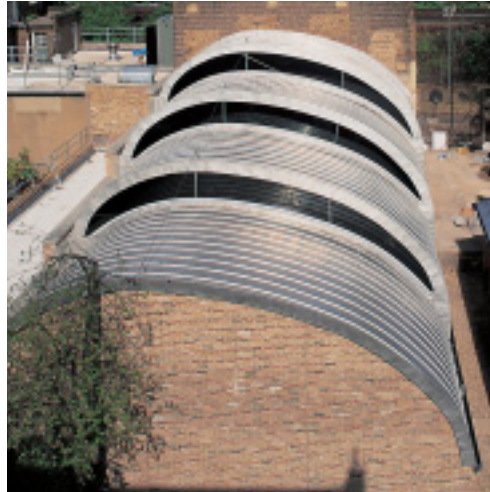
Stainless steel is used for the outer skin of this unusually shaped roof.
