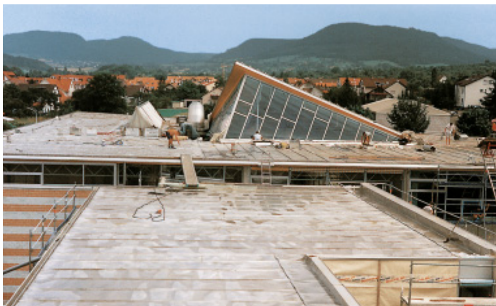
The seam-welded stainless steel roofing before planting (right) and afterwards (far right).
