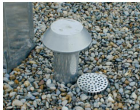
Stainless steel gully in a loaded flat roof next to a ventilation outlet and a chimney cladding in the same material
