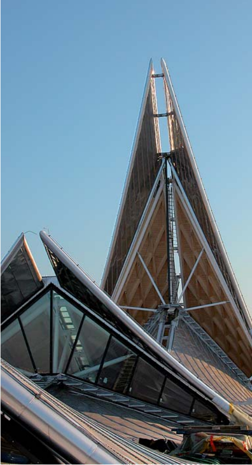
By offsetting the small and the large roof cones, space is created for north-west-facing skylights.
