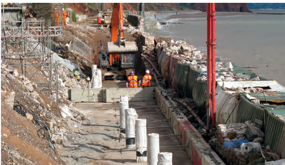
Grip Bar stainless steel tie bars being installed in the base of the new concrete sea wall at Dawlish. © Network Rail
