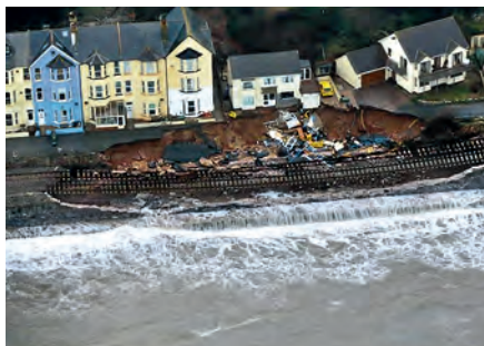
The train track in Dawlish was left suspended in mid-air after storms battered the sea wall in February 2014. © Network Rail
