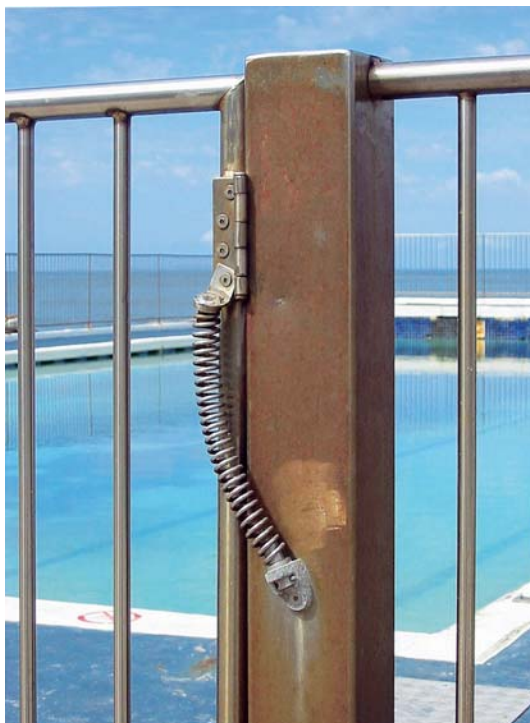
Figure B The contrast in appearance between the gate and support post is due to stainless steel chemistry and surface roughness differences. The corrosion-free gate is Type 316 stainless steel and the post that is discolored by corrosion is Type 304 stainless steel. (Photo Courtesy of Australian Stainless Steel Development Association)
