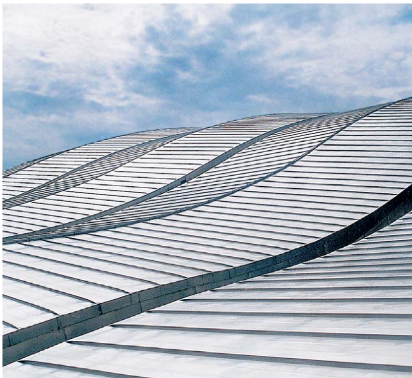
Figure B This photo shows the unique roof design and the corrosion-free performance of the Type 316 stainless steel. (Photo Courtesy of Ewing Cole, Photographer: Erhard Pfeiffer)
