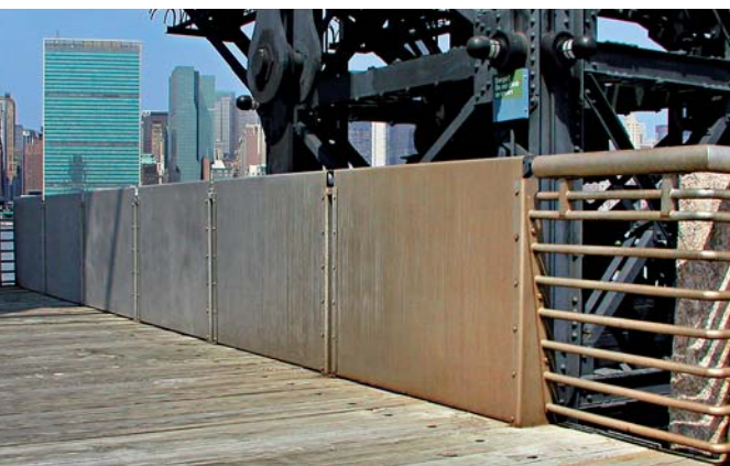
Figure C The Type 316 stainless steel has performed well on the piers. The exception is the splash zone, where there is discoloration caused by corrosion staining (right side of image).
